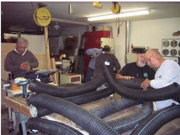
The Woodmere team of Pepe Corello and Frank Gagliano thread nylon rope through the drilled holes and secure the pipe with sprockets designed from recycled material.
